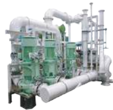
C.F.W Pumps Unit
